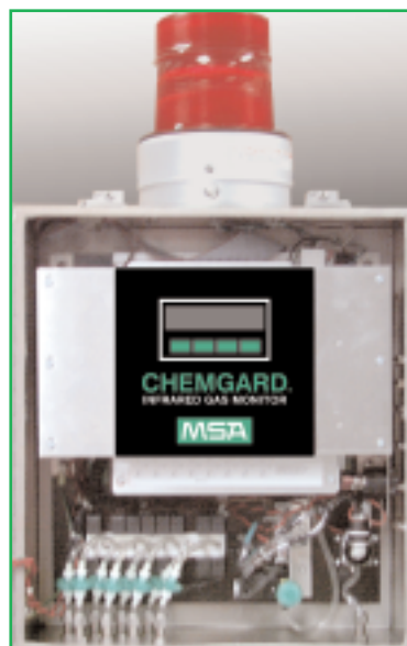
Figure 2. Interior of housing showing Chemgard Monitor with multipoint sequencer
